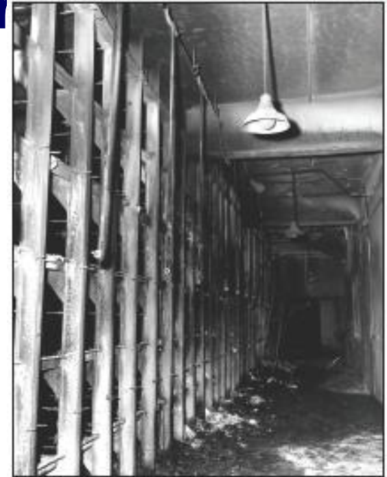
In 1969 spontaneous combustion in a glovebox in Building 776 started a fire that spread through the filter plenum.
